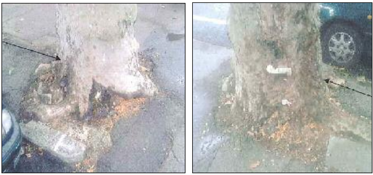
Photos of subject tree (arrow indicates location of sensor 1). Visually trunk appears to be in reasonable condition however when tapped with a nylon mallet, sounded partly hollow. Picus test, along with wood samples, confirms extensive damaged/decayed wood.
